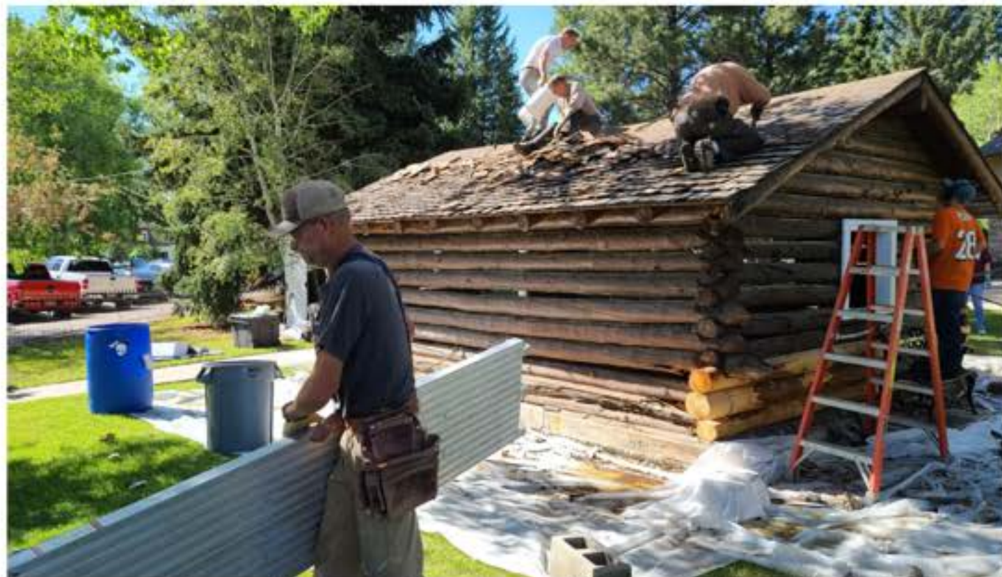
LPM Volunteers and Davis Logworks crew removing old shingles from the Marshall Schoolhouse.
